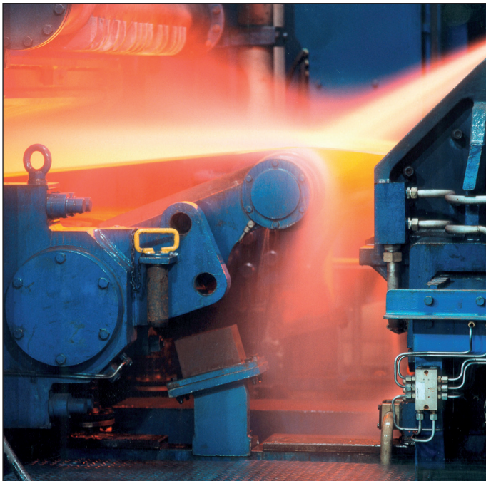
Siemens will supply the work roll cooling and anti-peeling systems for stands F2 to F4. Photo courtesy of ThyssenKrupp AG
