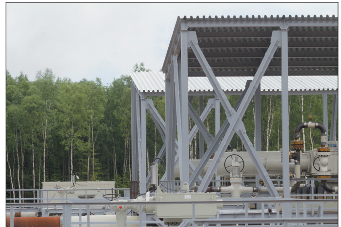
Onshore facilities located 1.5 kilometres from the shoreline include pig traps as well as isolation and emergency shutdown valves. Installation of equipment was completed in June. Photo courtesy of Nord Stream AG
